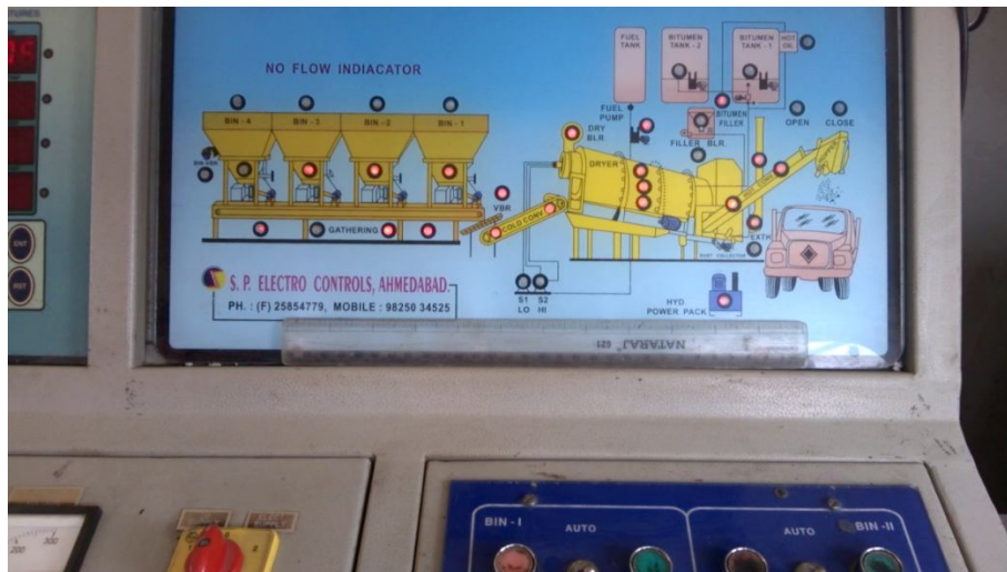
Fig. 3 Main display screen of SCADA control panel (Actual Photograph on site)
