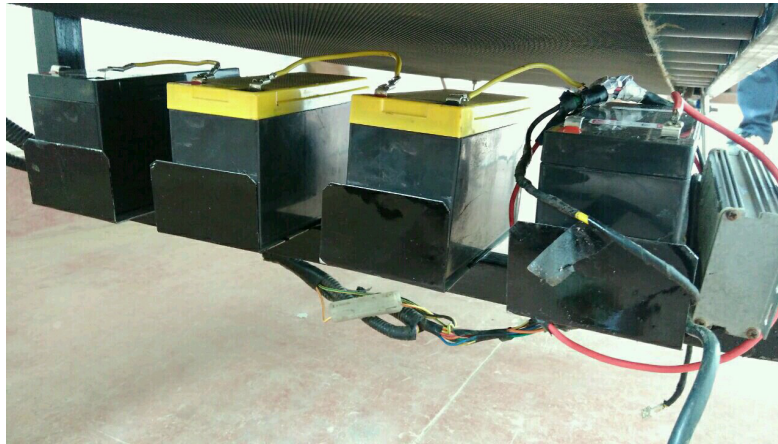
Fig. 4.4.1 Battery – Controller unit
